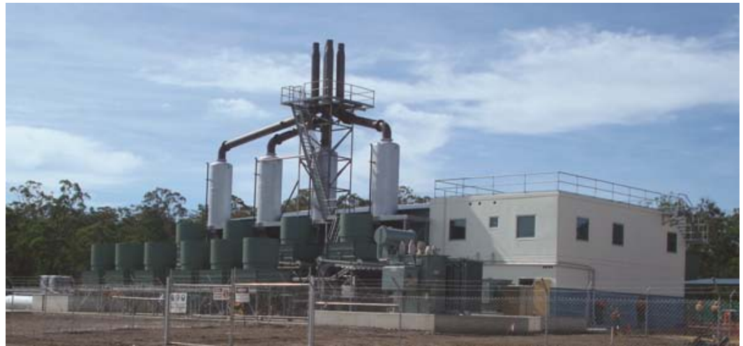
5MW Power Station at Bloodwood Creek, Queensland.
