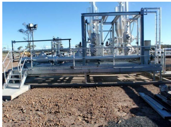
Panel 2 Knock out pots and access platforms
